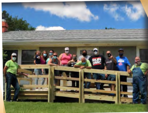
Servants at Work volunteers are happy to have finished a ramp for a mobility challenged resident.
